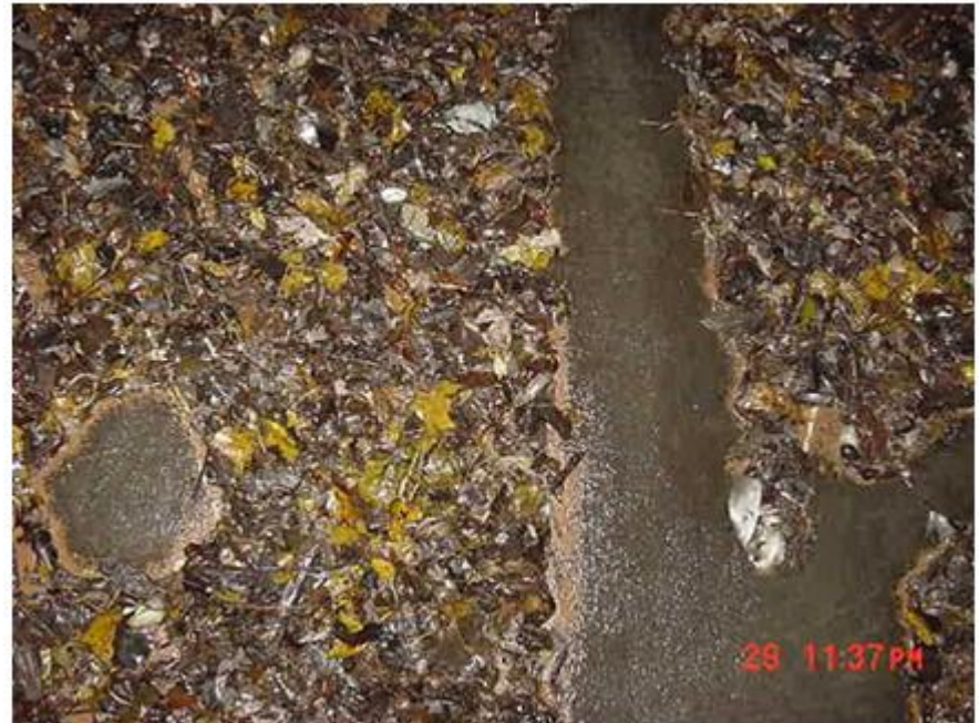
Debris in condenser from typical "thru flow screen" due to debris carry-over
