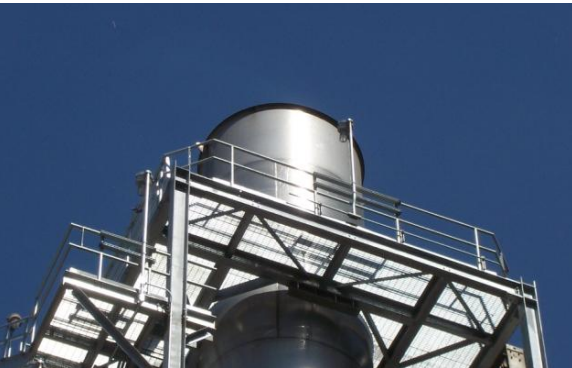
Wet ESP Power On
