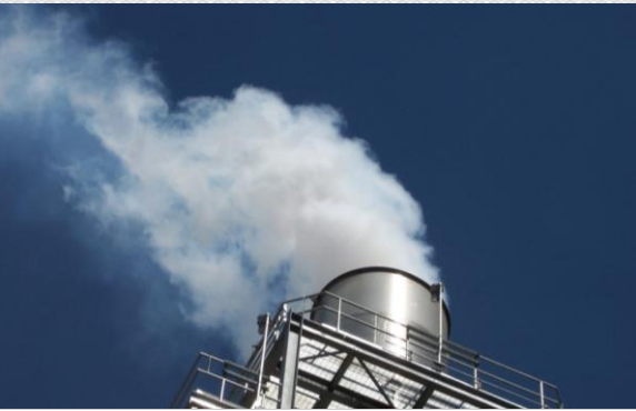
Wet ESP Power Off
