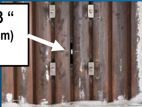
Slotted Opening in Membrane
