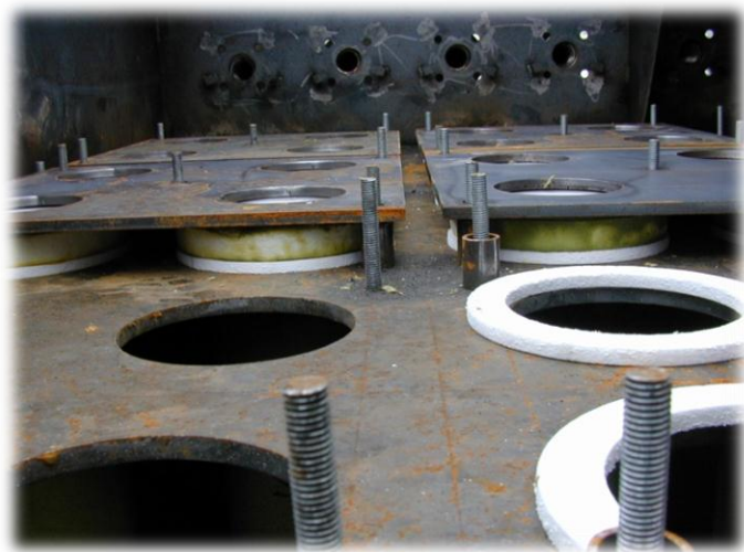
Tube sheet, seals and filter elements
