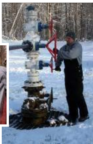
Injection well head
