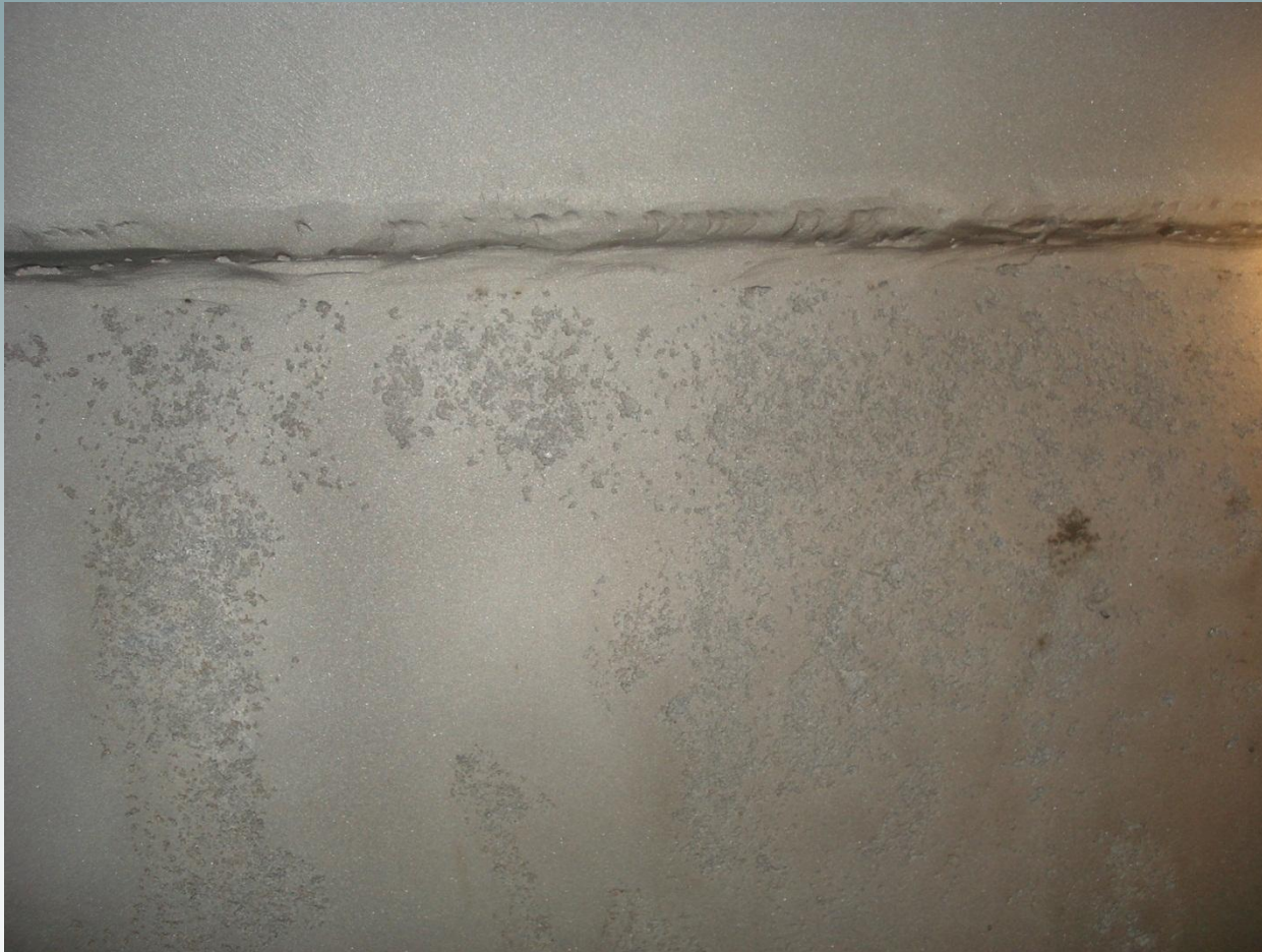
Crevice corrosion of duplex steel absorber wall adjacent to weld
