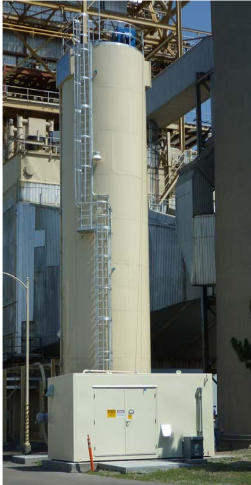
Albemarle ACI Silo System with Optional Controls & Blower Building
