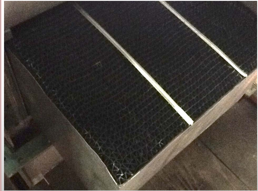
Top View of Module Removed for inspection
