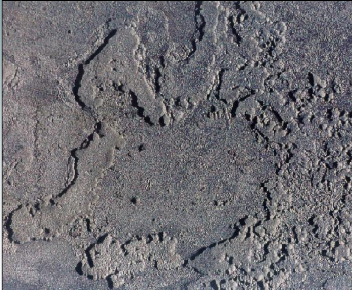
Corrosion under ash deposit
