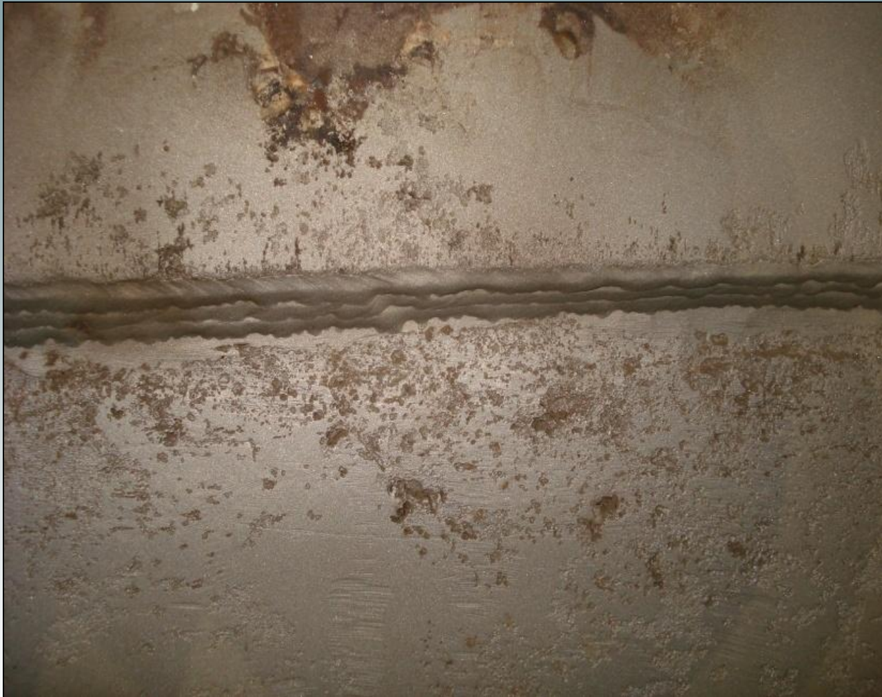
Corrosion of duplex steel absorber vessel. The nickel alloy 625 weld was not attacked.
