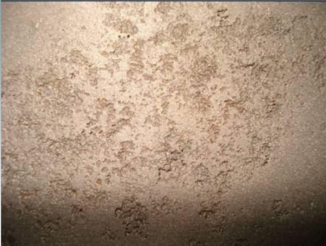
Crevice corrosion of duplex steel absorber vessel wall located well away from weldment
