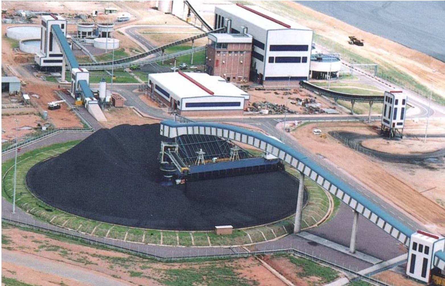
Stacker (slewing and luffing) with Bridge Reclaimer
