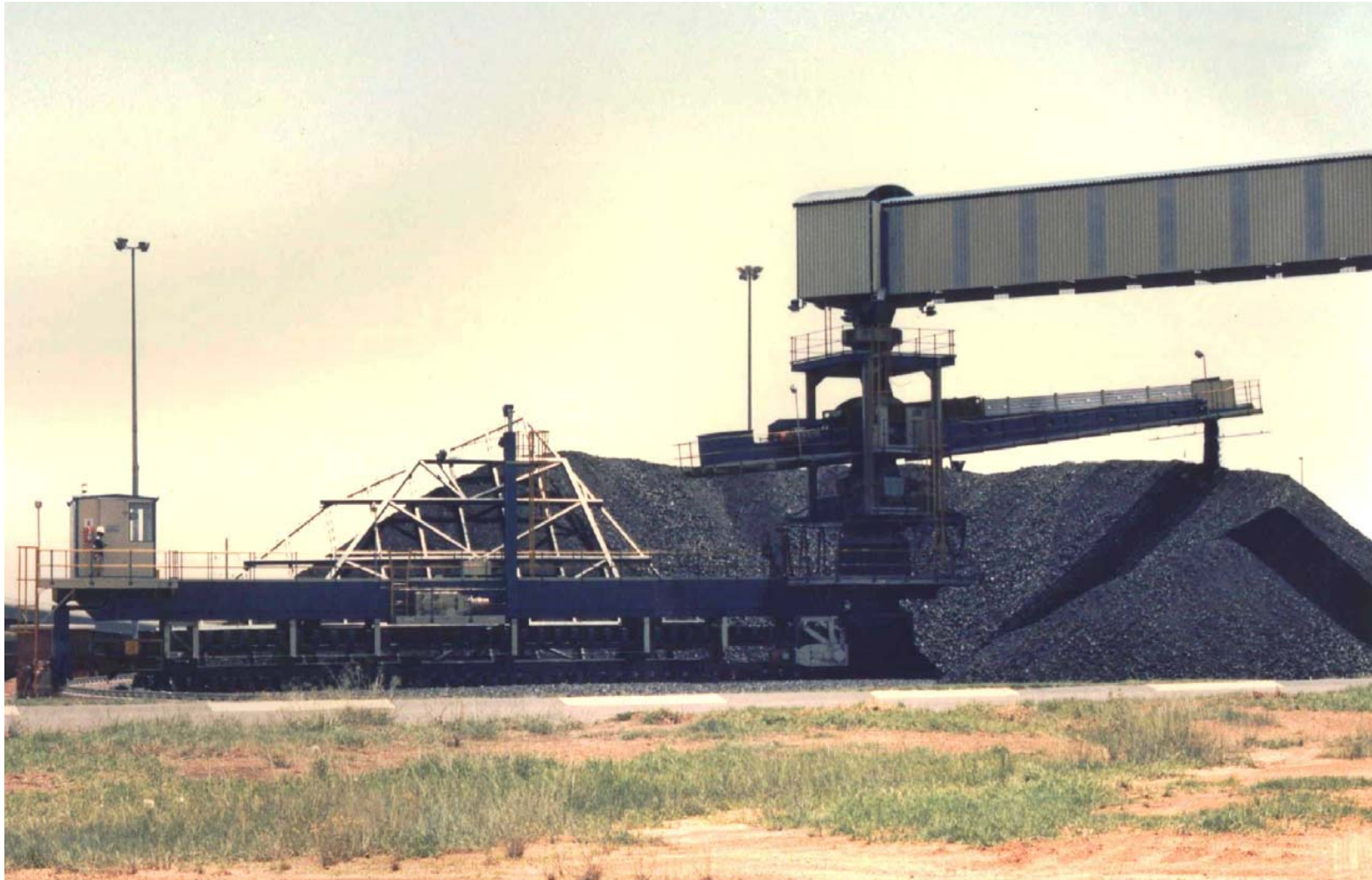
Stacker (slewing and luffing) with Bridge Reclaimer
