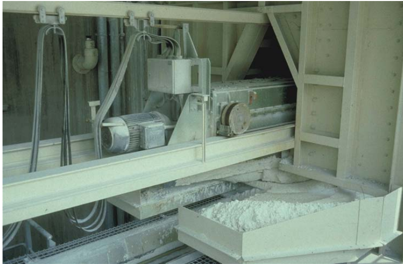
RDM-BL 3000; 11 kW 90 t/h FGD-gypsum Idstein - Germany
