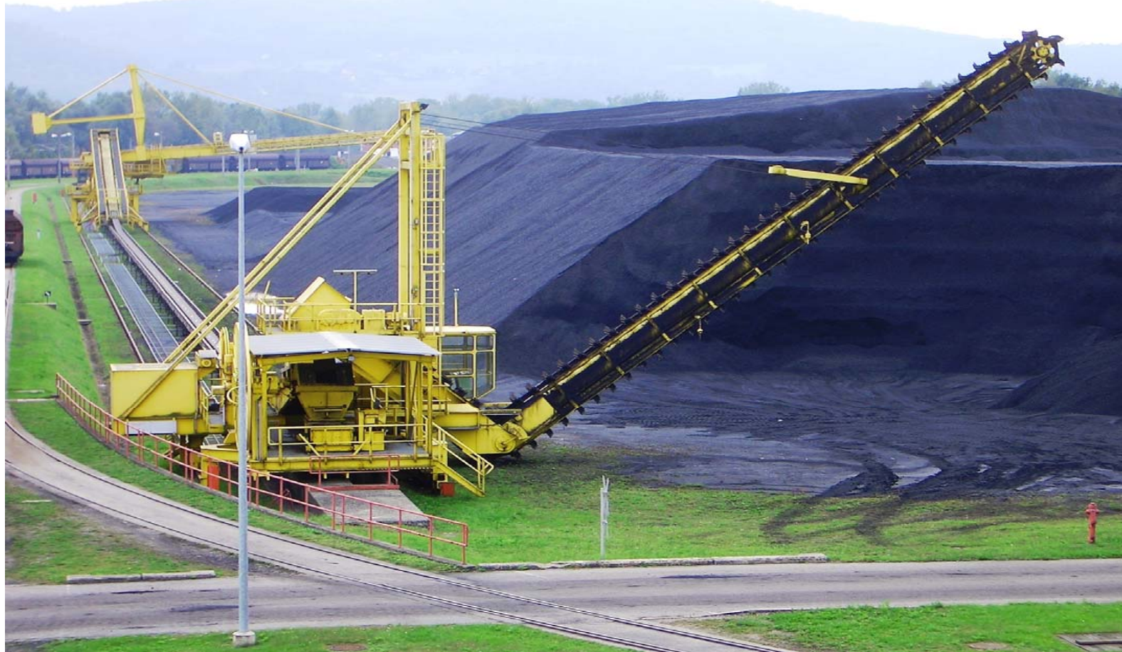
Cantilever Reclaimer (discharge via drag trough)
