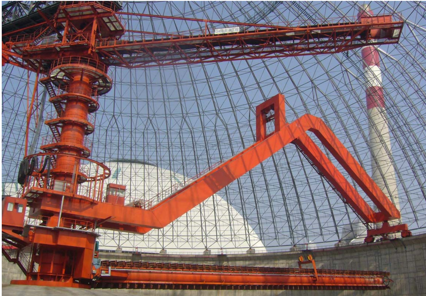
Stacker (slewing) with Semi-Portal Reclaimer (slewing and luffing)
