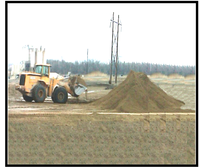
Dewatered Bottom Ash
