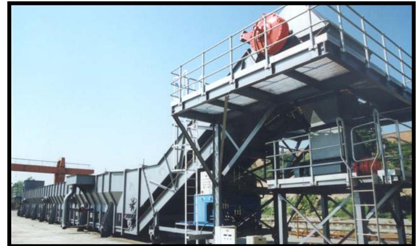
TO – A SUBMERGED SCRAPER CONVEYOR
