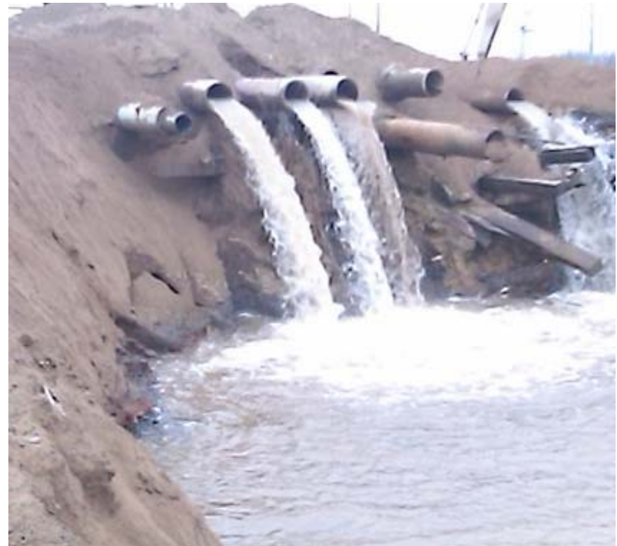
Bottom Ash discharged to an ash pond
