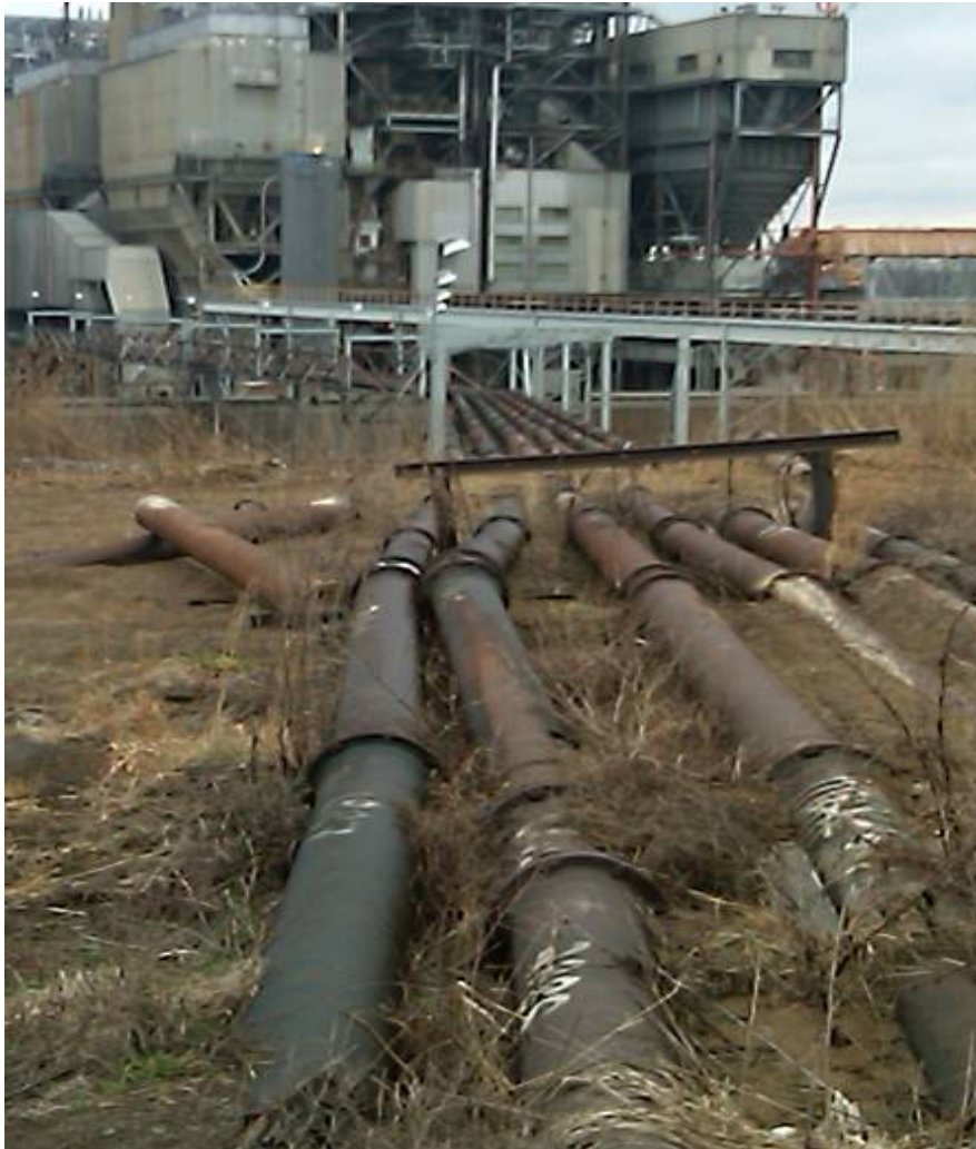
Typical Bottom Ash Slurry Piping
