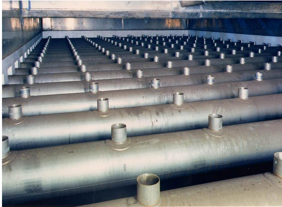
AL-6XN Slurry Piping for NIPSCO Baily Station
