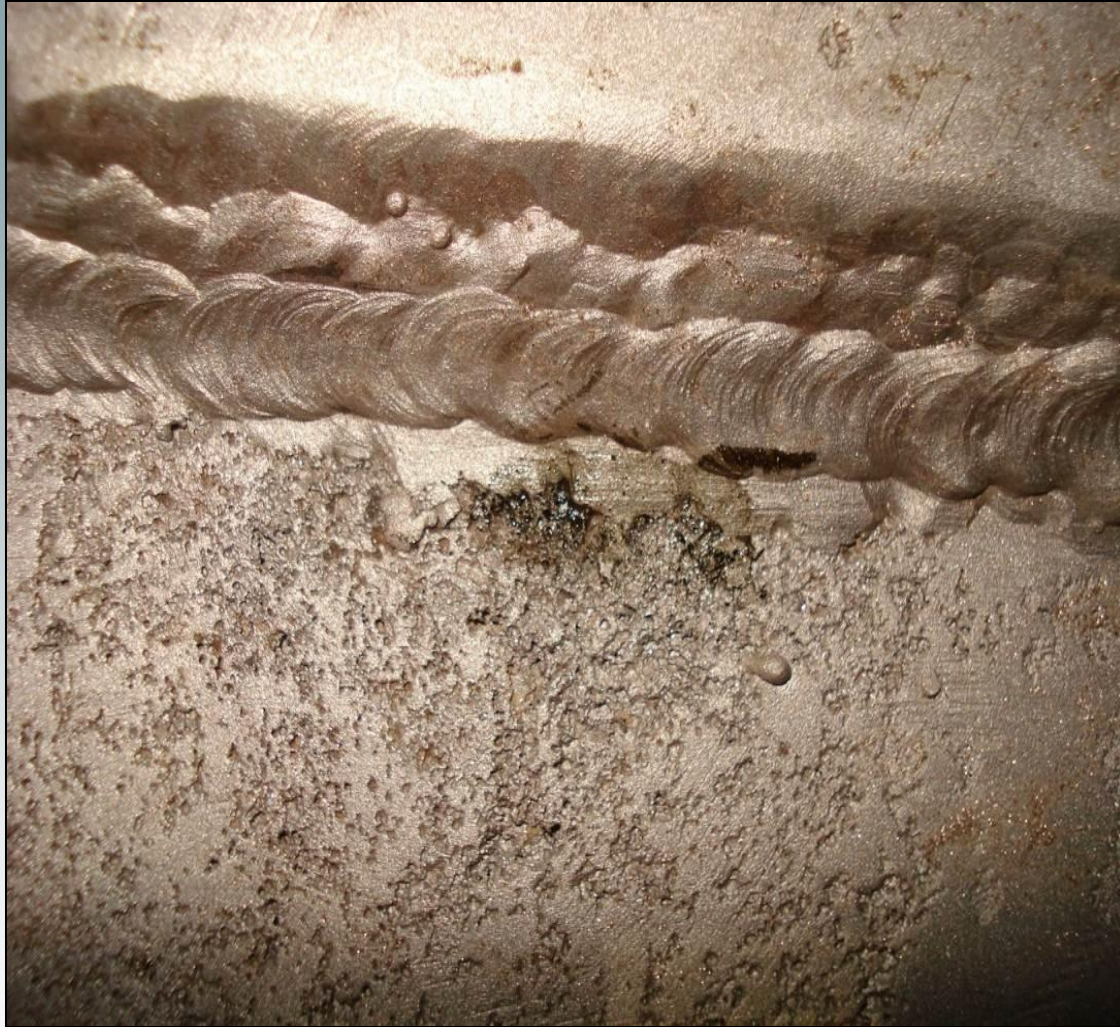
Attack of 2205 duplex steel absorber. Bottom plate is original construction. Upper plate is repair. Weld is alloy 625.
