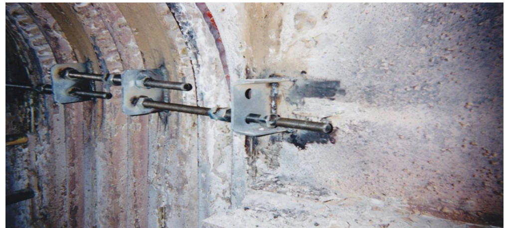
E) Internal liners removed. Old metal EJ becomes new flow liner. Add control rods for increased metal "EJ LINER" life.
