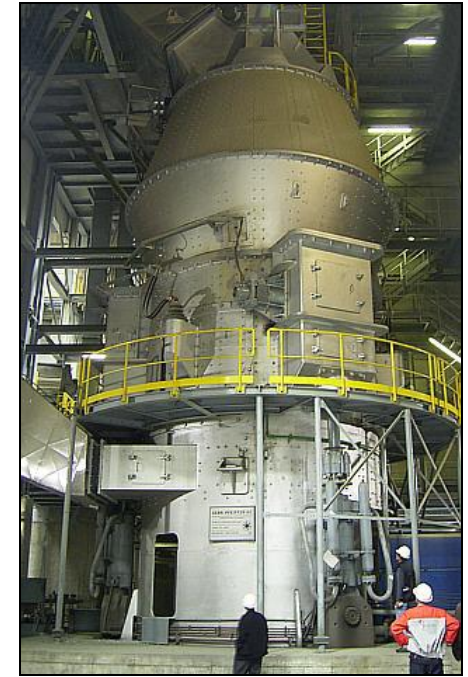
MPS cement mill
