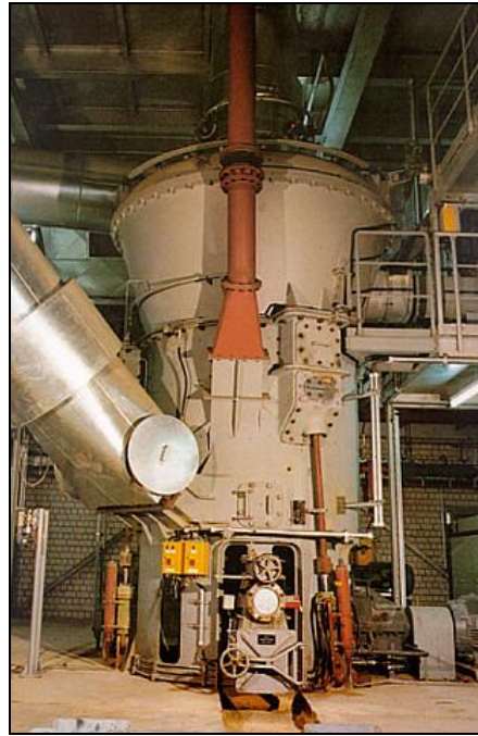
MPS coal mill
