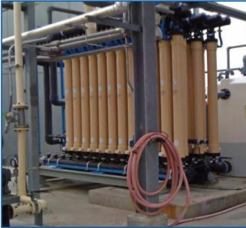
Pall Aria MF-System (136 m 3 /h; 600 gpm)
