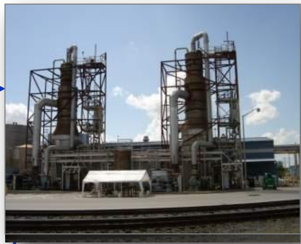
2 EVAPORATORS / BRINE CONCENTRATORS (2x0.7 MW)
