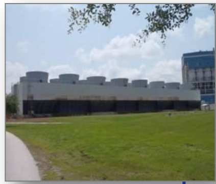
COOLING TOWER (4-7 COC)
