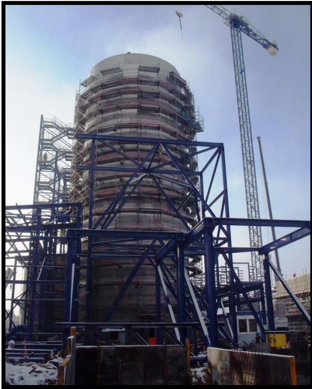
Combined Heating and Power Plant | Pulawy, Poland
