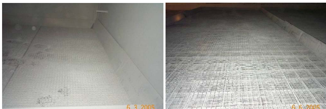
Figure 18 Typical FCC catalyst fines build-up (left) and catalyst layer after cleaning
