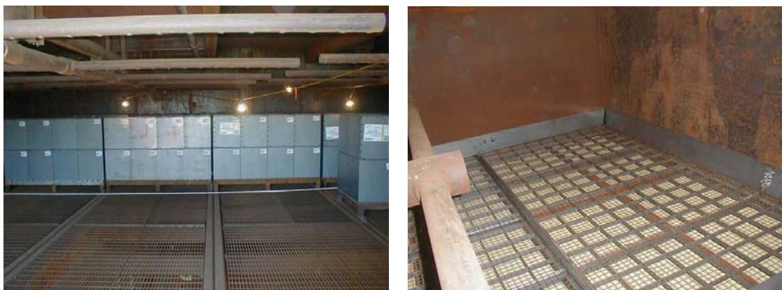
Figure 20 Each catalyst layer has 40 Haldor Topsøe VE422AA catalyst modules (left). Dust deflectors along the reactor wall prevent FCC catalyst fines from collecting in the space between the walls and the modules
