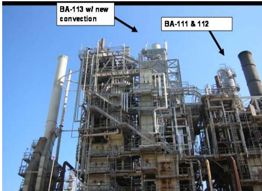
Figure 10 Additional convection sections placed on top of the existing heater of the ethylene plant at Chevron Phillips, Cedar Bayou, Texas, USA
