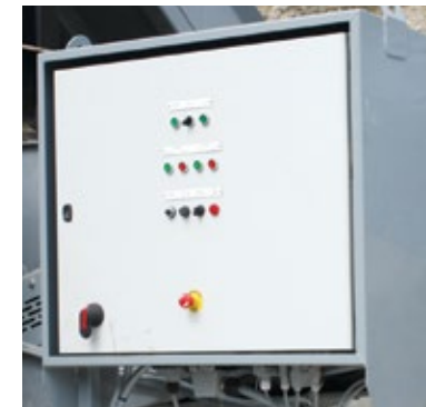
H12 Feeder Control Panel
