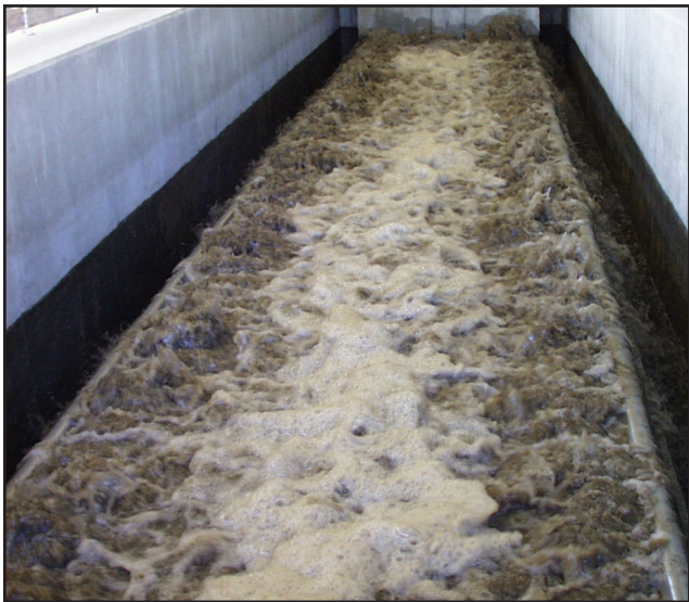
Combined air/water, sustained, sub-fluidized backwash cleans the media, with backwash water consumption as low as 2% of the forward flow.
