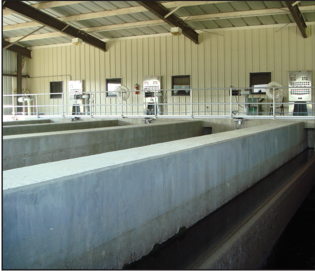
Special, deep-bed biofiltration system is credited with key contribution to utility's continued compliance with state total nitrogen limits, despite ongoing rapid growth in service demand.
