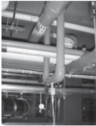
Figure 4. Photo depicting sample drain configuration.
