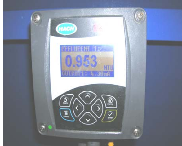
Clari-DAF system effluent registers below one NTU.
