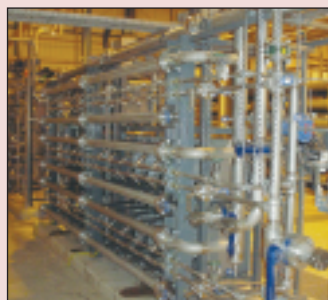
CDI system skid
