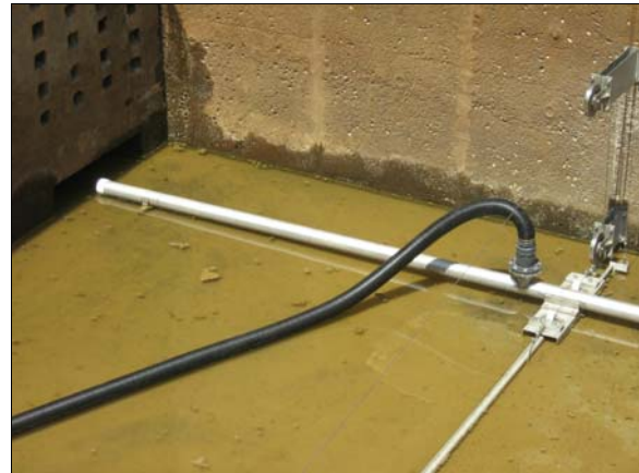
Installation of the CT2 submerged sludge collector is completed in the basin in preparation for operation.
