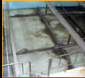
SONGJEON WATER TREATMENT PLANT, WONJU, KOREA The Songjeon Water Treatment Plant, operated by the Korean Water Resources Corp, obtains raw water from the Hoeng-Seong Lake.
