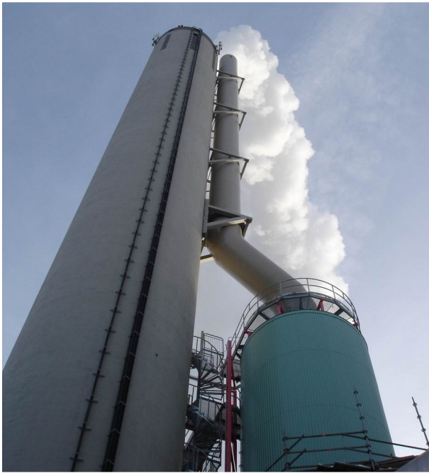
Picture 2 Two-Stage Scrubber/Cooler
