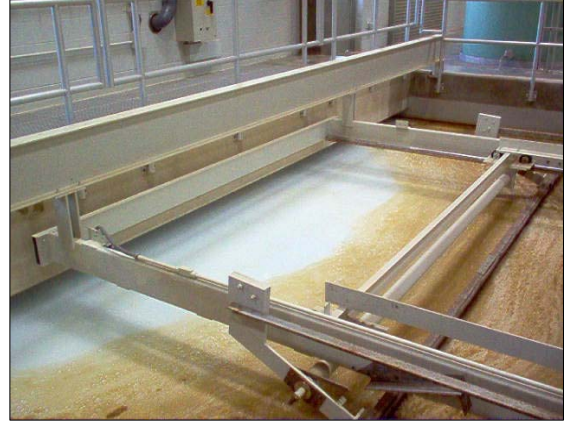
The Clari-DAF system at work.
