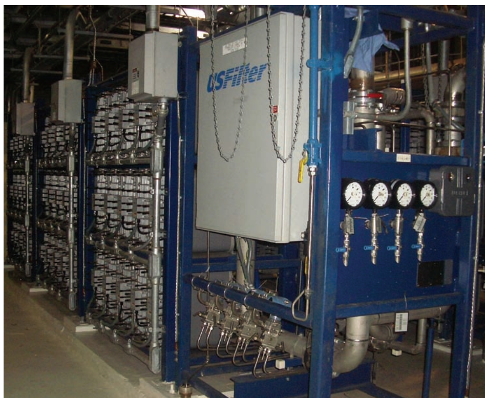
Figure 1: 1500 m 3 /h CEDI System at East River Generating Station (1 of 10 skids).
