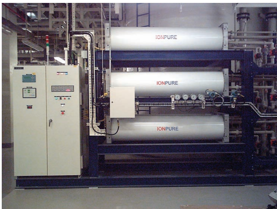
Figure 3: 70 m 3 /h CEDI system using stacked-disk modules.
