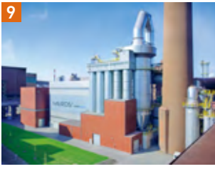
9 Sinter Plant Equipped with Waste Gas Recirculation (Meros)
