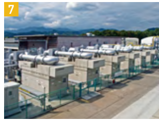
7 Highly Efficient Gas Engine Power Plant
