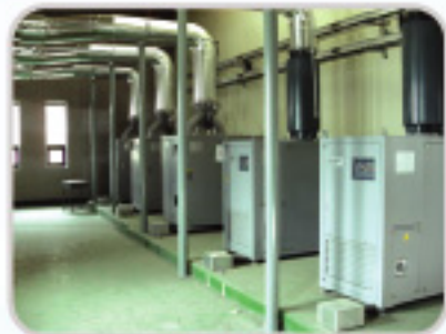
Sewage treatment center in Uijeongbu
