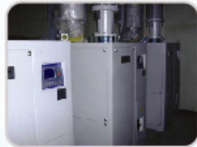
Sewage treatment center in Ulsan
