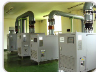
Sewage treatment center in Cheongju
