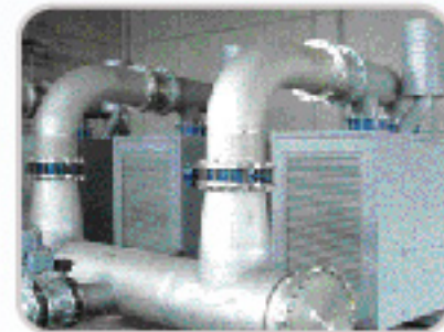
Sewage treatment center in Ahsan
