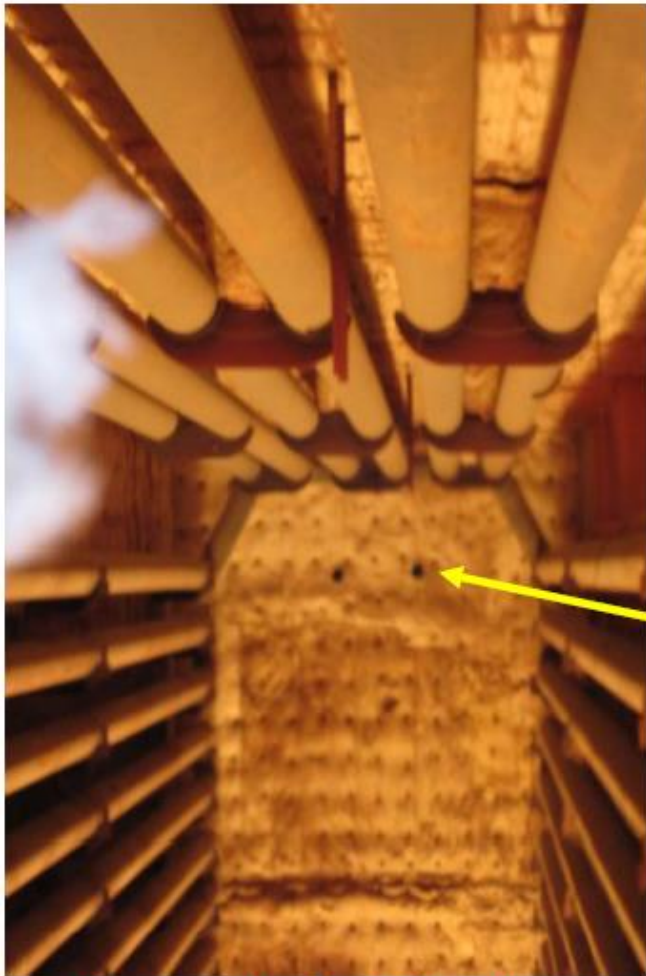
Furnace Radiant Section
