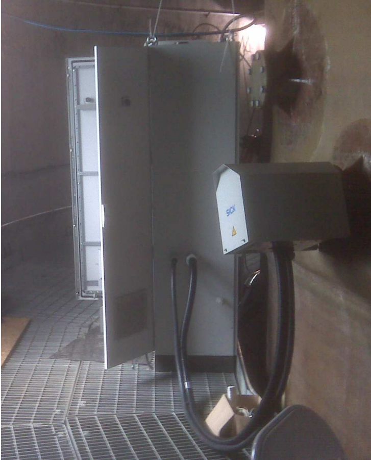
Photo 2: Installation of the MCS100 E HW at the stack with heated filter probe.
