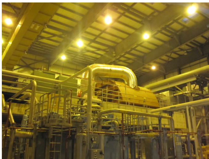
Figure 11: High Pressure Sodium Lighting in Turbine Building
