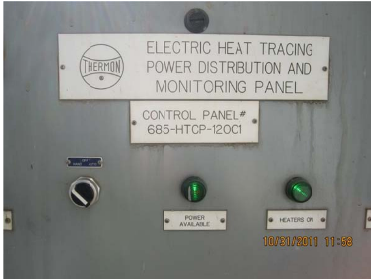
Heat Trace Panel with Heaters On While Ambient Temperature was 50 - 60°F
