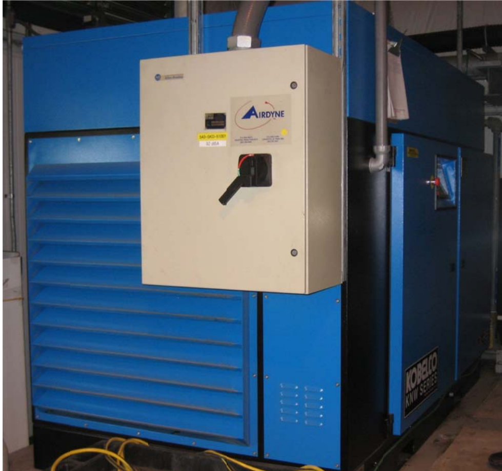
Existing Oil-free Load-unload Rotary Screw Air Compressor
