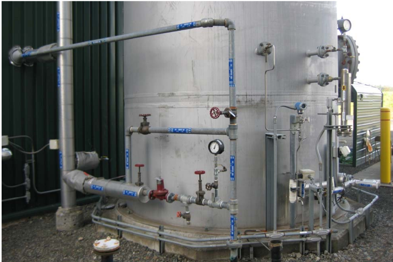
Compressed Air Receiver with the Priority Valve Feeding the Plant Air Lines
