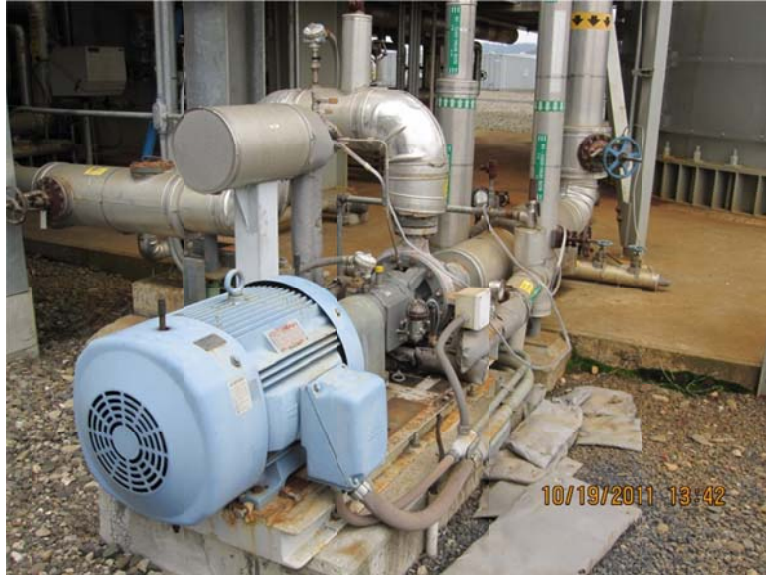
Low Pressure Economizer Recirculation Pump
