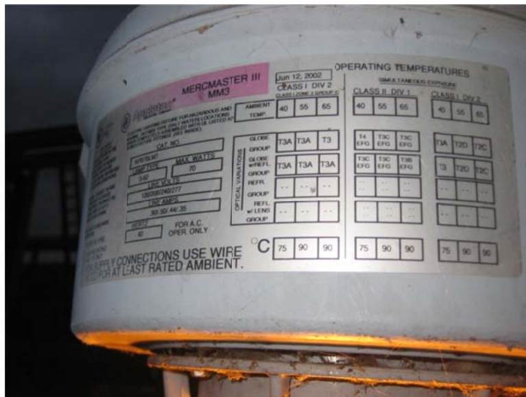
Outdoor Light Nameplate Information
