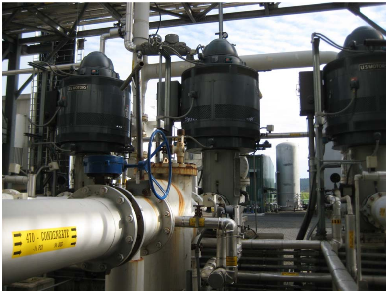
Existing 450 hp Turbine Style Condensate Pumps (1A, 2A, and 3A)
