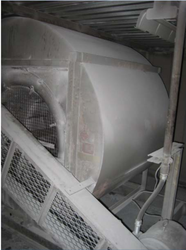
Typical fan of 14 fans in bank
