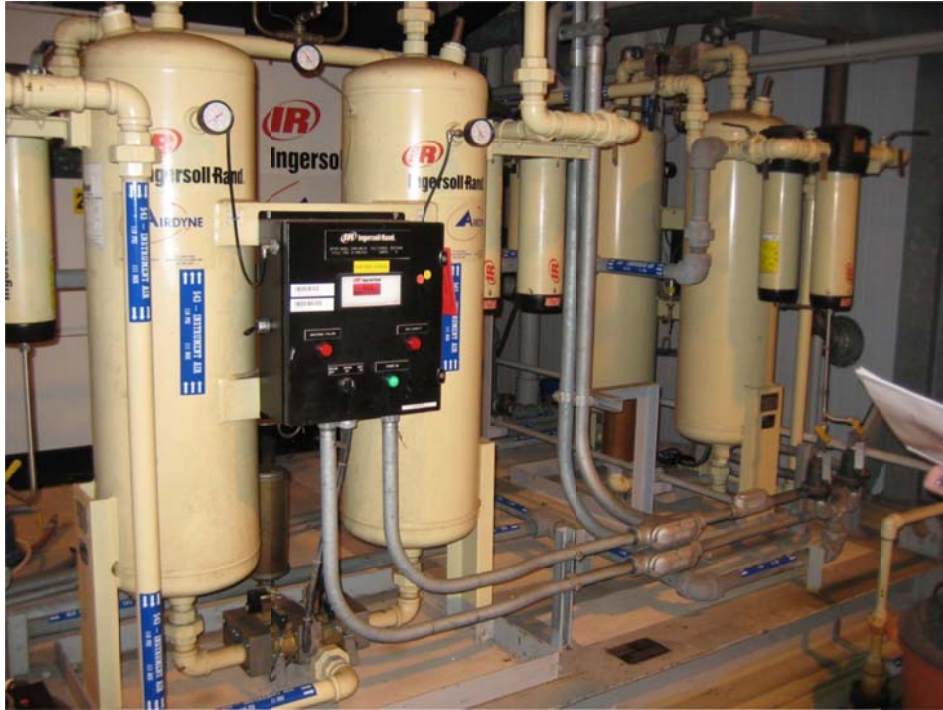
Two Dual Tower Ingersoll-Rand ThermoZorb 300 Heatless Air Dryers
