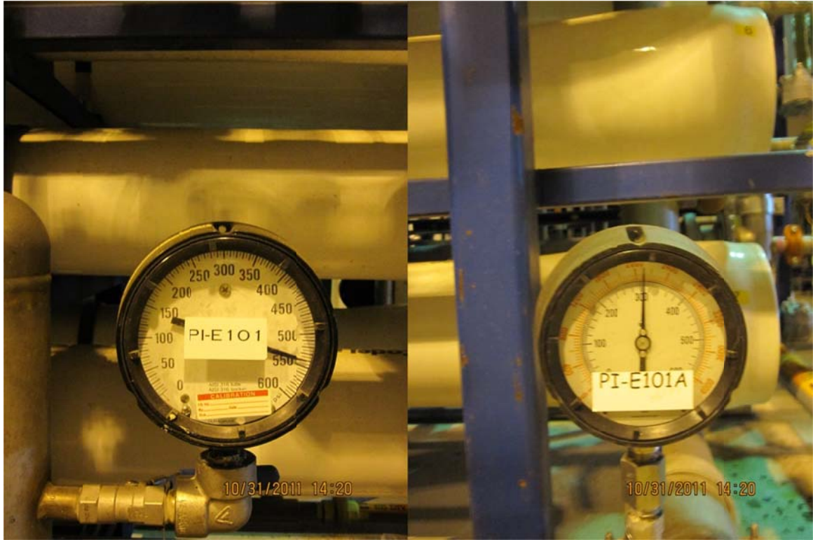
First Pass Discharge Pressures Before (left) and After (right) Valve
