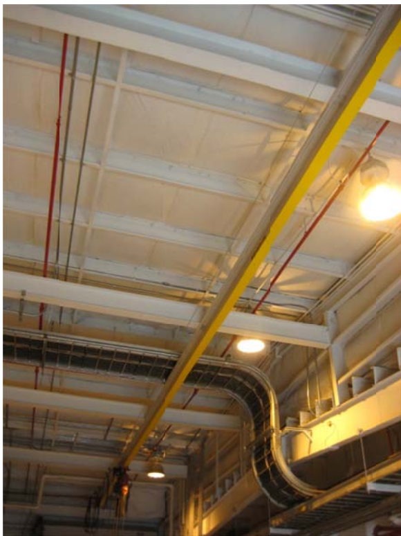
Indoor High Pressure Sodium Fixtures
