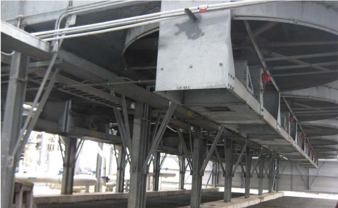
CCW Fans and Underside of CCW Heat Exchanger
