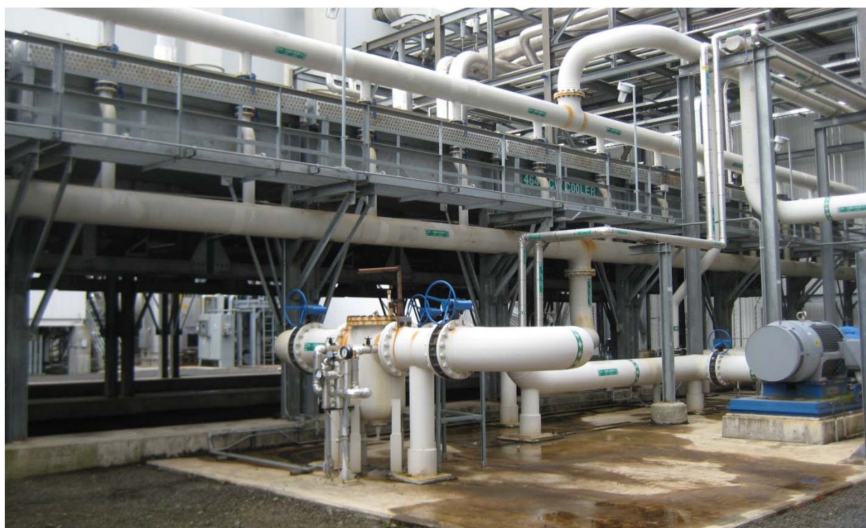
Figure 8: Closed cooling water system with cooler on the left and one of the two 550 HP pumps on the right
