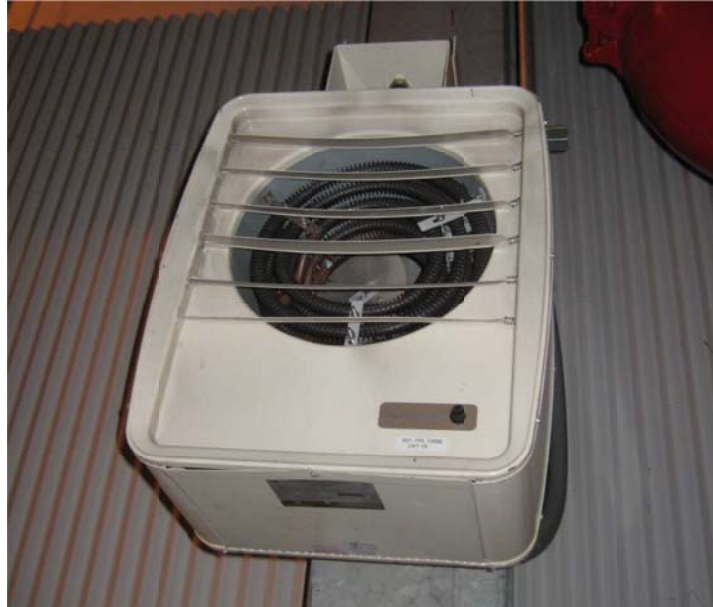
One of the 20 kW Space Heaters in the Turbine Building
