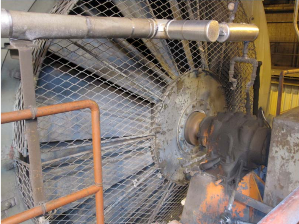
Inlet Vanes on Forced Draft Fans
