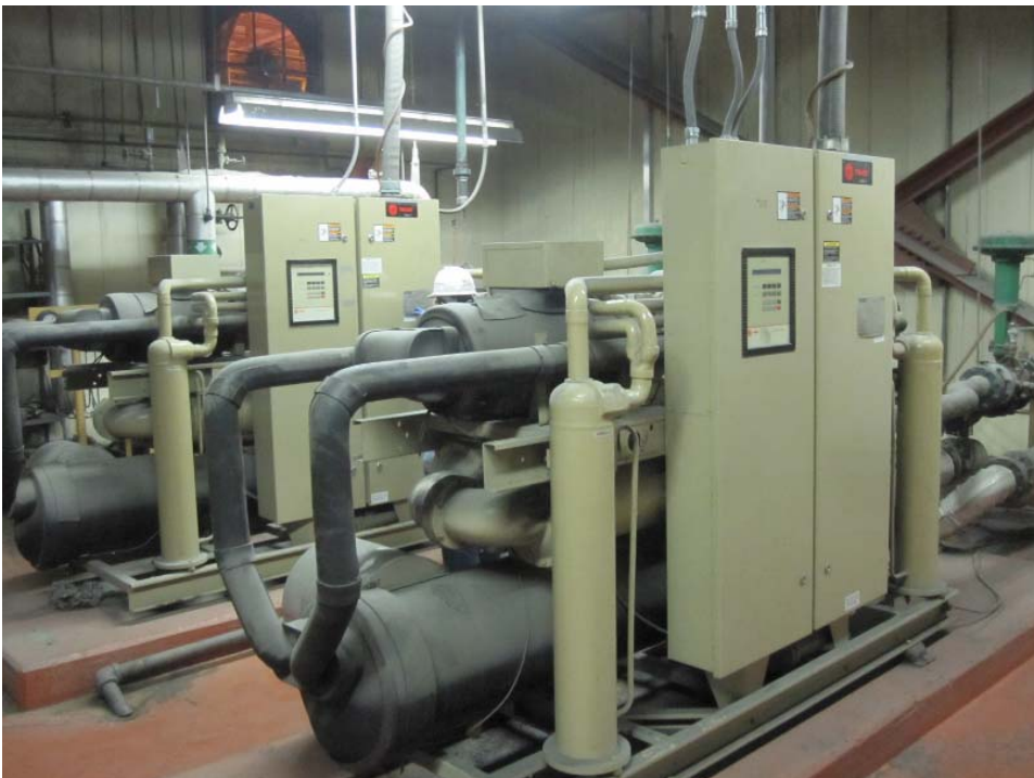
2 Chillers for control room
