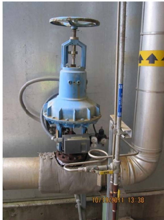
Gutted Temperature Control Valve Downstream of LP Economizer Recirculation Pump
