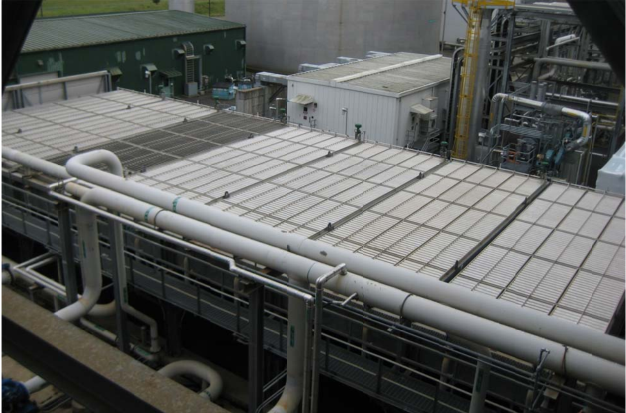
Louvers above CCW Heat Exchanger and Fans
