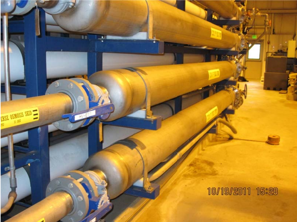
Reverse Osmosis Pumps
