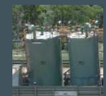
Alternative liquid fuel handling facility at Fishermans Landing plant Photo: CAPL
