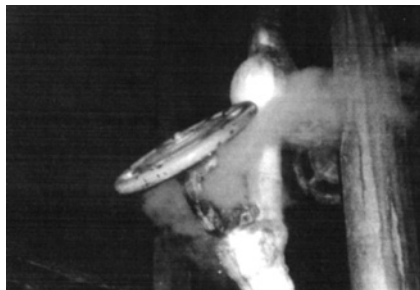
Continual stem leaks from globe valves allows plant efficiency to decrease and maintenance costs to rise.
