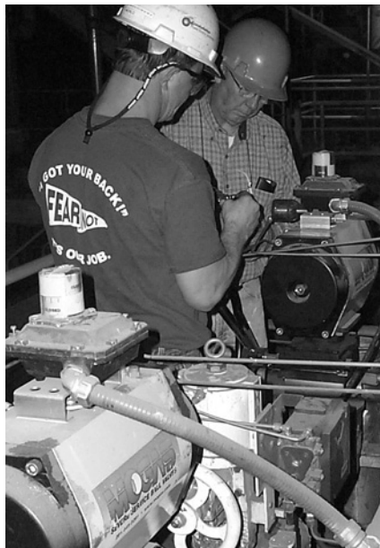
These four, 2-inch GEN-X MOGAS ball valves are handling Cold Reheat Isolation in a coal-fired plant.
