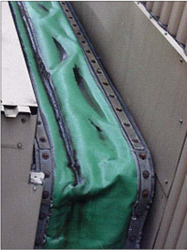
Figure 9 Economizer bypass expansion joint.
