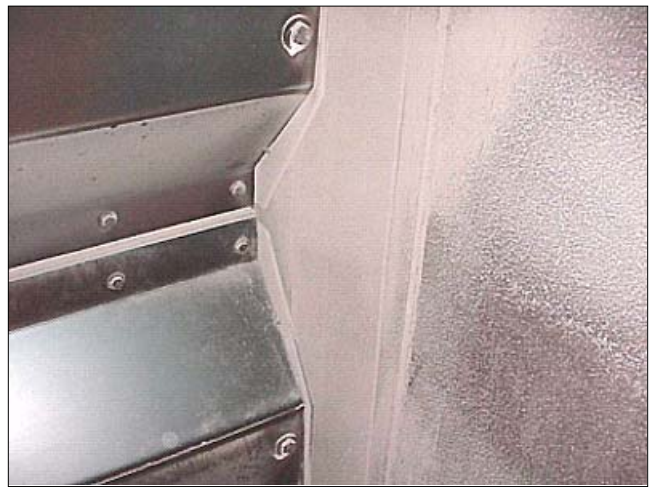
Figure 8 SCR bypass damper.
