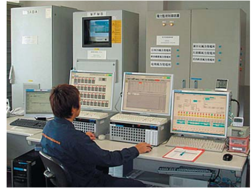
Central control room
