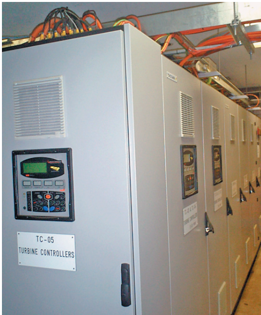
CENTUM CS 3000 control system cabinet
