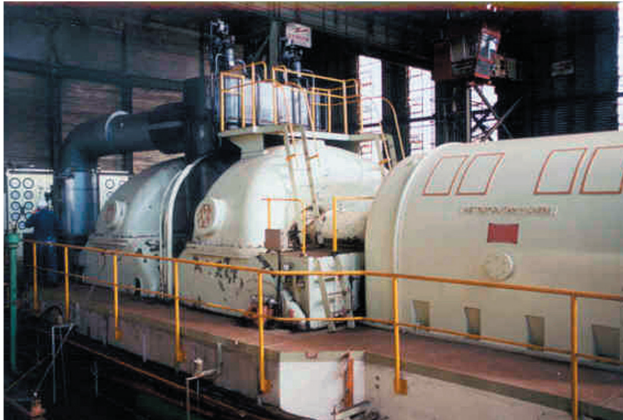
Low pressure condensing turbine generator
