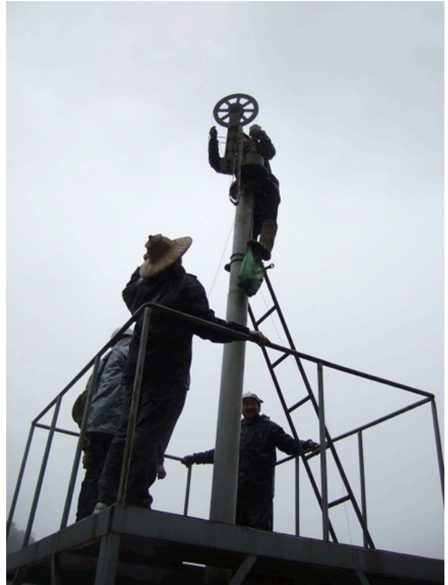
Right – Insertion of FBG temperature probe and fiber optic cable into the thermal well
