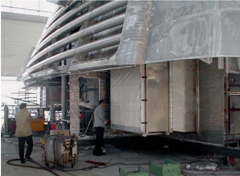
A view of the ship's funnel with filter modules mounted at the sides
