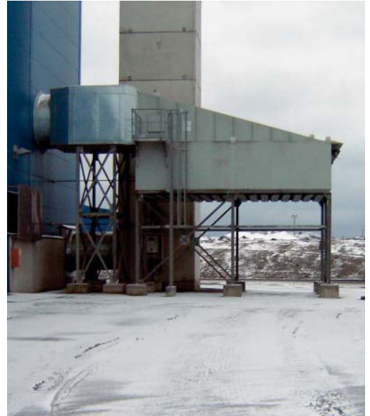
Sideview of the outdoor intake air filter housing
