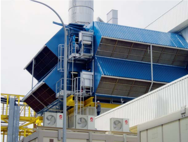
3-sided air intake filter system of the combined-cycle power plant (Philippines, SEA)
