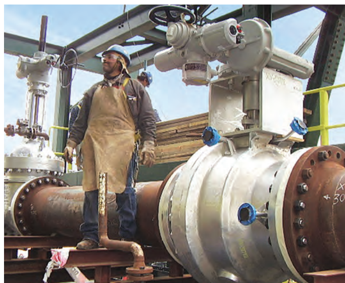
NPS 30 (DN 750) overhead vapor valve prior to insulation.
