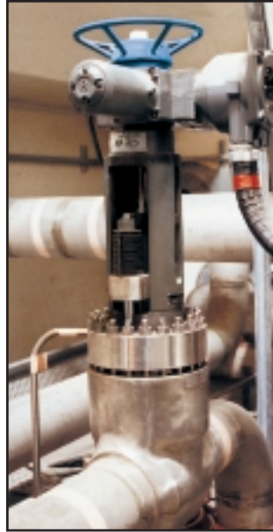
A Velan bolted bonnet valve in a PHT Transfer System.
