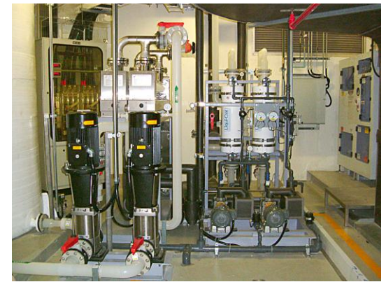
Second Stage Liqui-Cel Polishing System for CO 2 and O 2 Removal
