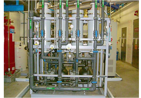
First Stage Liqui-Cel System for CO 2 and O 2 Removal
