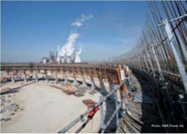
4 The Neurath lignite-fired power plant in Germany will be the world's biggest after its completion in 2010. The picture shows the construction site of one cooling tower. One Sulzer pump will feed each of the two 1100-MW boilers.
