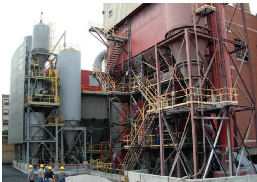
After being satisfied with the performance and reliability of the first dry scrubber (right), Virginia Tech officials opted for the same technology and installed a second system (left) 10 years later.
