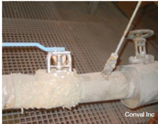
4. Ball valve for main-steam drain isolation service replaced an ineffective gate. Body is of F91 material
