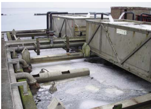
▲ Whatever the water-handling application - water supply, cleaning shellfish, cooling, seed harvesting or packaging - today, all of the approximately 35 pumps used in this P&D facility are supplied by ITT brands including Lowara, Vogel, Flygt and Hydrovar.
