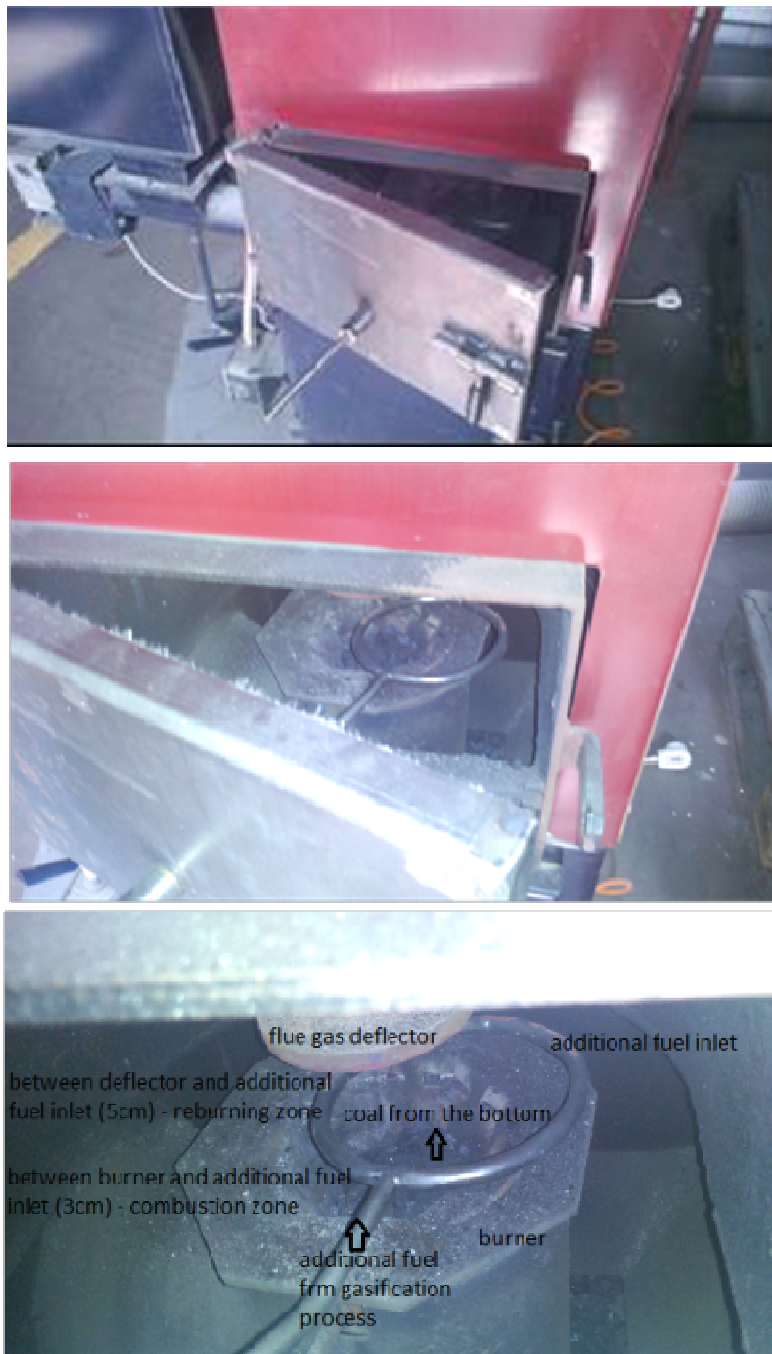
Fig. 6. Boiler modifications - additional fuel inlets
