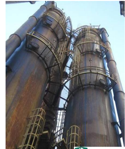
800 TPD (2 trains) commercial CO 2 capture system treating slipstream from coal-fired boiler MEA Solvent Standard Flow Scheme
