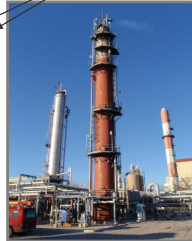
150 TPD commercial CO 2 capture system treating slipstream from coal-fired power plant MEA Solvent Standard Flow Scheme
