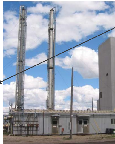
Boundary Dam Pilot 5 TPD Pilot plant treating slip stream from coal-fired power plant RS-2 and MEA Solvent TKO™ Flow Scheme
