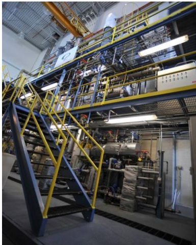
International Test Center 1 TPD Pilot plant treating exhaust from gas turbine RS-2 and MEA Solvent TKO™ Flow Scheme
