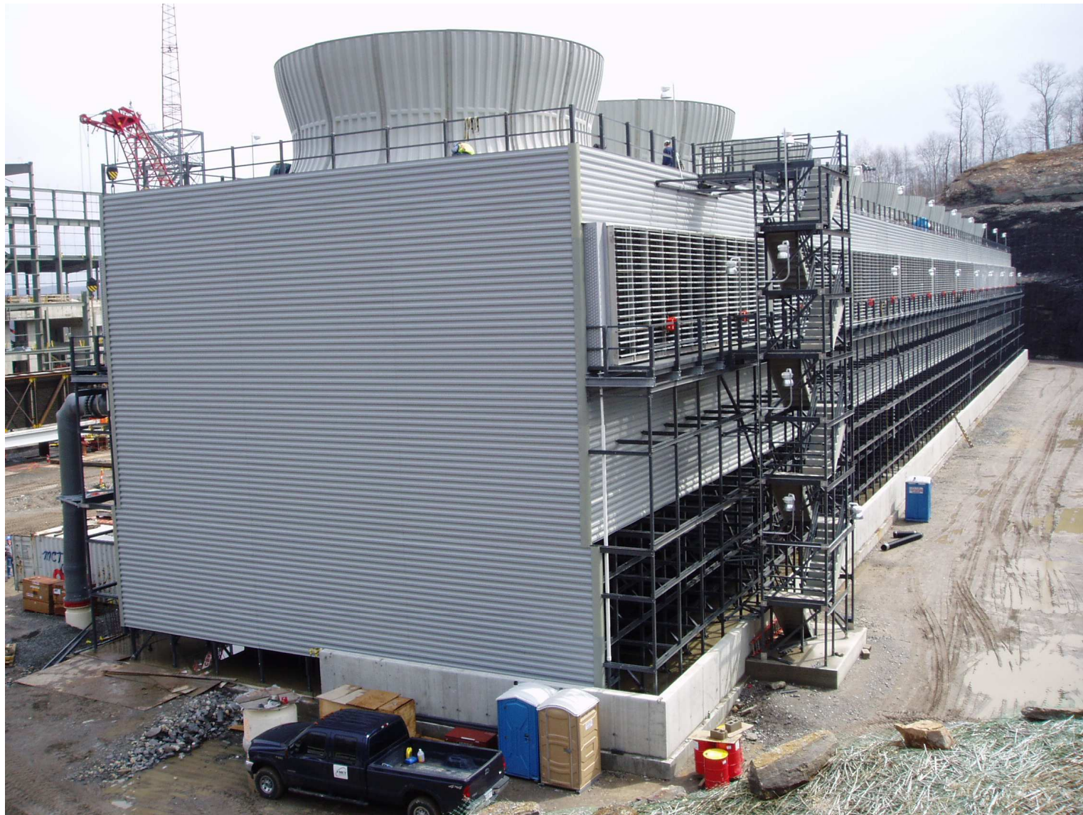
Counterflow Wet Dry Cooling Tower
